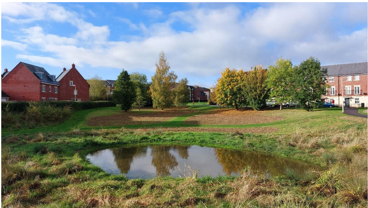
Streamside SuDS (sustainable urban drainage) Pond
